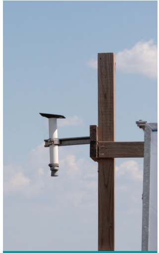
(See story on left) Real-time flood sensor installed in flood-prone region.
