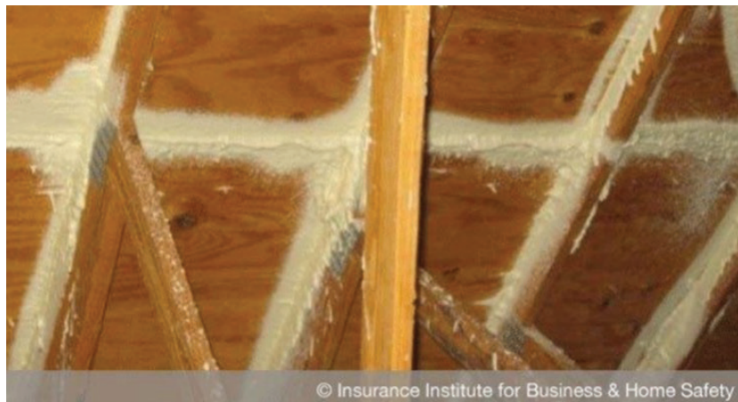
Figure 3-6. Spray Foamed Attic Source: IBHS
